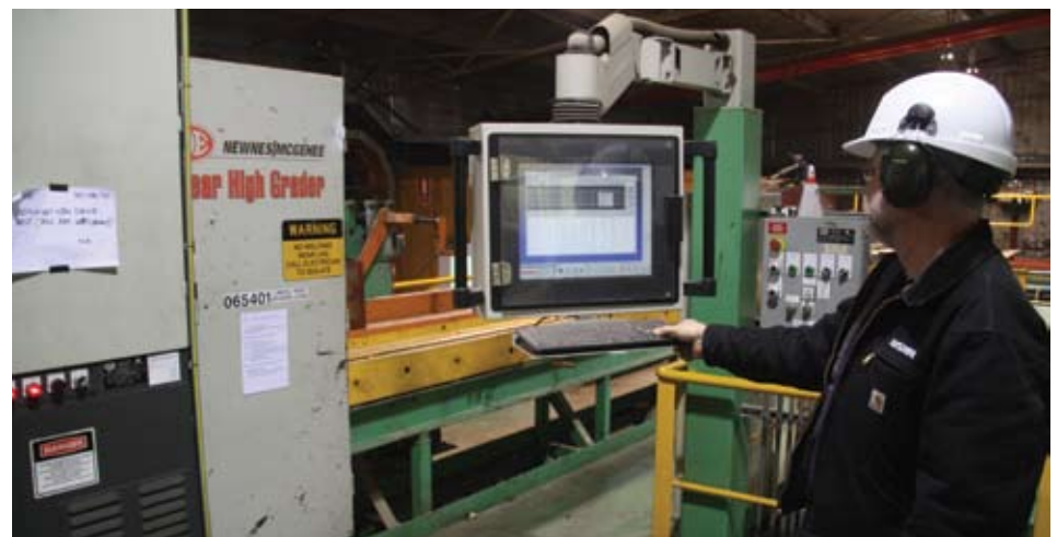
USNR technician, Mark Allert, adjusts parameters on Wespine's Lineal High Grader (LHG) automated grading system during an on-site visit. The LHG was installed at this site in 2005.
